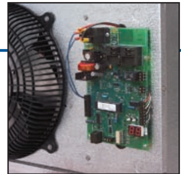
The Master Controller Reverse Cycle control panel with housing removed.
